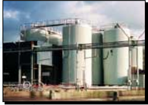
Level measurement on storage tanks
